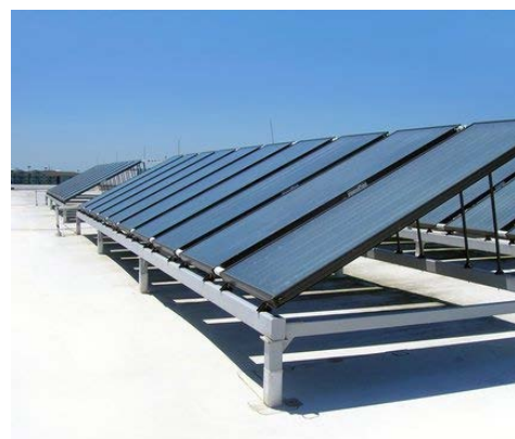
Figure 5. Commercial SWH system – IKEA Orlando
