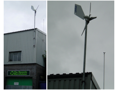
Figure B.9. An Ampair “600 W” micro-turbine. The average power generated by this micro-turbine in Leamington Spa is 0.037 kWh per day (1.5 W).
