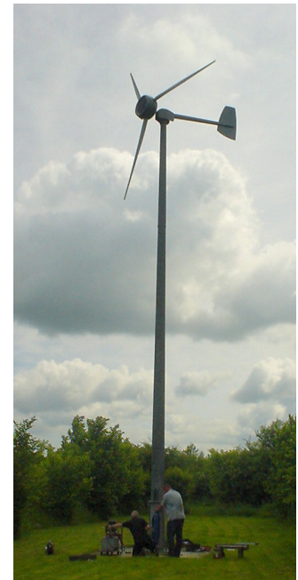
Figure B.10. A 5.5-m diameter Iskra 5 kW turbine [ www.iskrawind.com ] having its annual check-up. This turbine, located in Hertfordshire (not the windiest of locations in Britain), mounted at a height of 12 m, has an average output of 11 kWh per day. A wind farm of machines with this performance, one per 30 m × 30 m square, would have a power per unit area of 0.5 W/m 2 .
